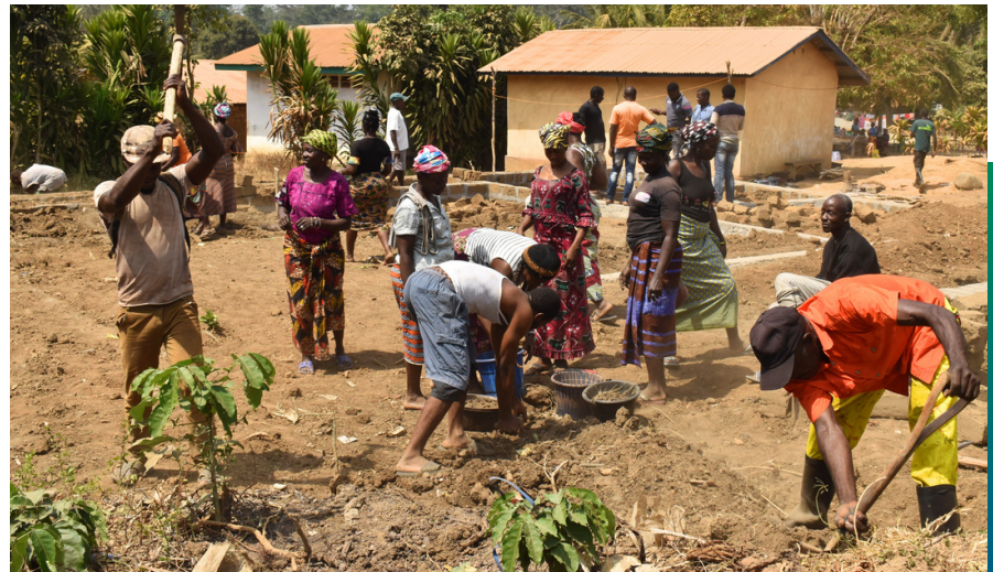
Gbeka and Maloma community members working together on construction for their Lead project
